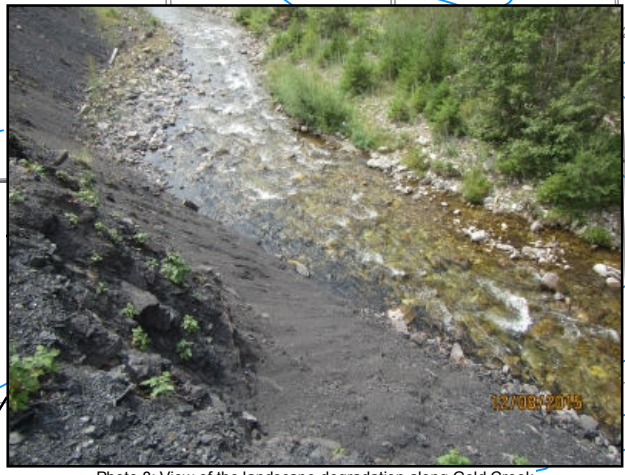
Photo 8: View of the landscape degradation along Gold Creek resulting from Legacy mining activity (July 2014).
