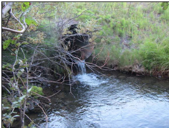
Perched culvert under Devon Road, Aug 2014.
